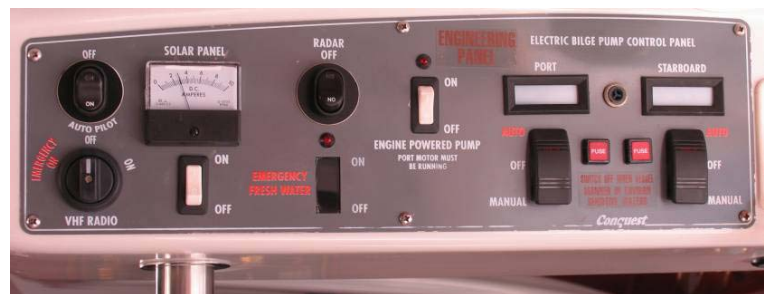
Figure 2.3 Engineering control panel with autopilot switch, vhf radio switch, solar panel charging meter, and bilge-pumping control switches.
