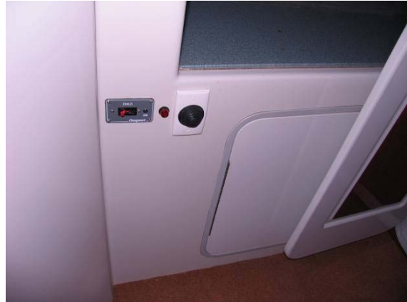
Figure 4.2 Holding tank pumpout control panel showing circuit breaker/switch on the left and push-button timer switch on the right
