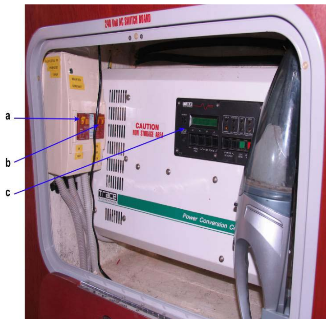
Figure 4.5 Inverter with circuit-breaker control switches for ship power (a), shore power (b) and menu selector buttons (c) to control the inverter functions (see text for details)
