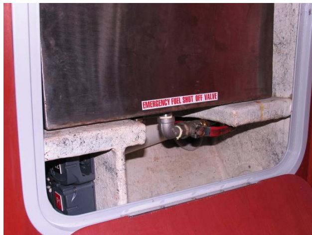
Figure 3.3 Diesel fuel tank in locker at aft end of port companionway showing fuel shut off valve.
