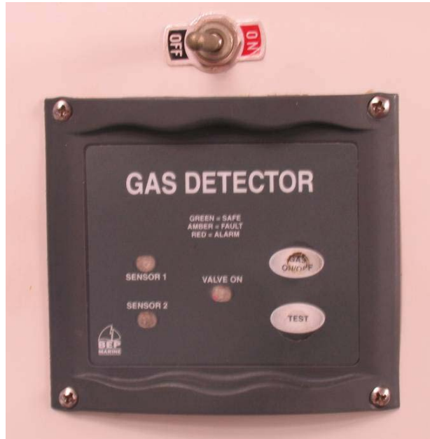
Figure 4.4 Gas detector and solenoid control unit (midships, in the centre of the saloon, mounted under the deck-head above the galley bench.
