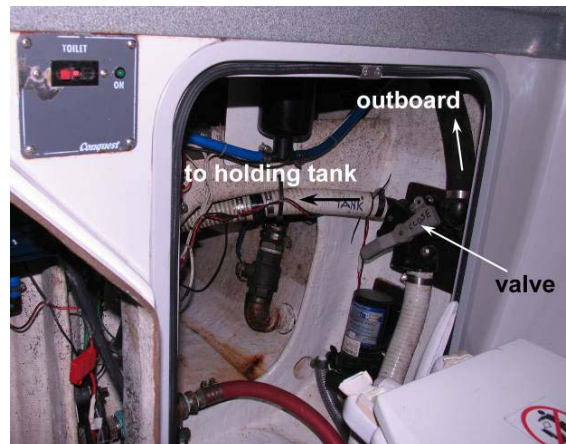
Figure 4.1 Valve to direct toilet discharge into holding tank or outboard. Note switch to turn on toilet pump controller in upper left of photo.
